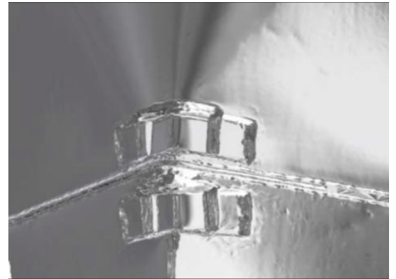
Processed scan of a crack damaged duct corner. The damage has been tried repaired by drilling crack end holes, grinding and welding the crack, and by welding on patches. The repair failed as both the repair welded crack and welded on patches cracked after a limited number of Start/Stop Cycles.
